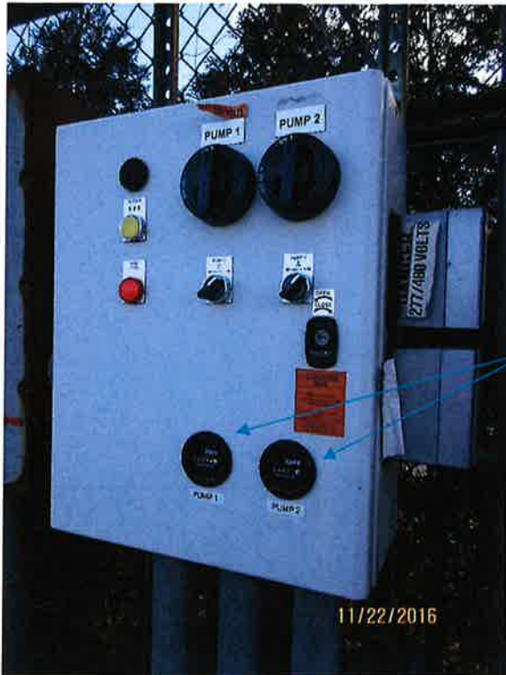
Photograph 1 – Pump run-time meters
