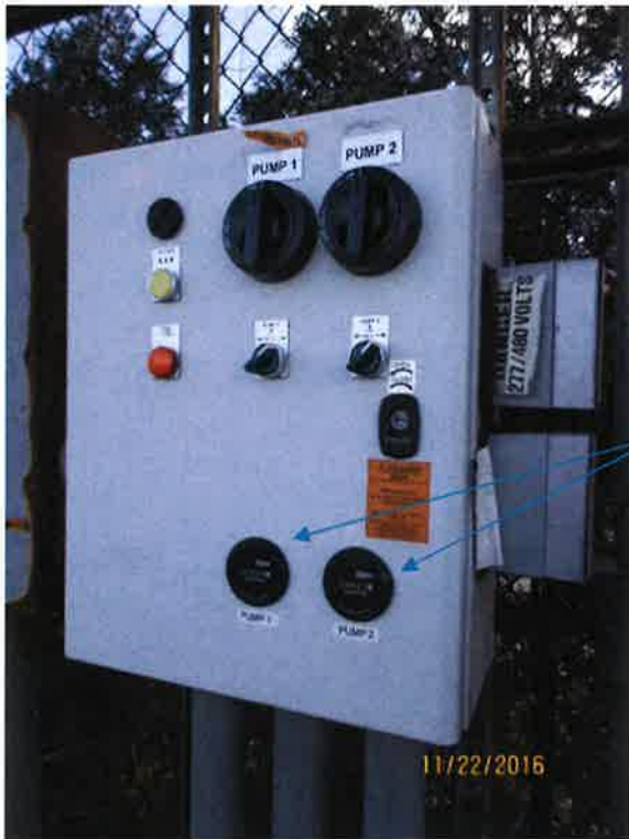
Photograph 1 – Pump run-time meters
