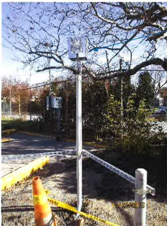
Photograph 2 – Solar powered wet sensor electronic housing
